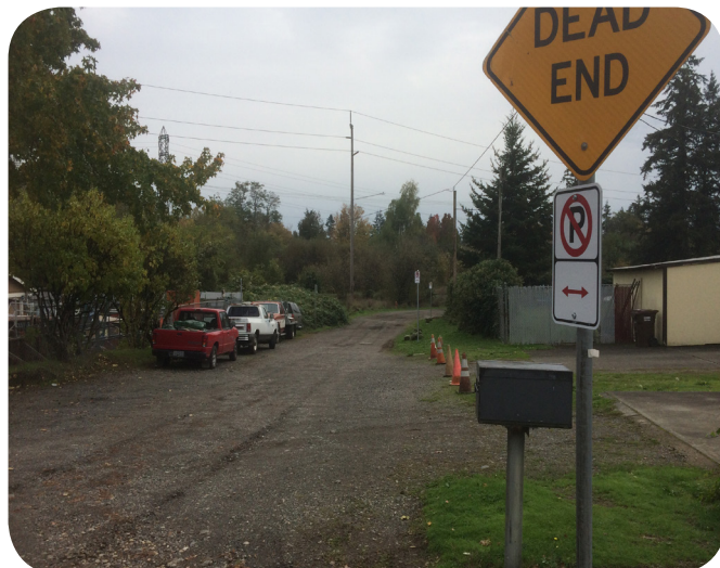
No pavement or sidewalks on an entire street.
